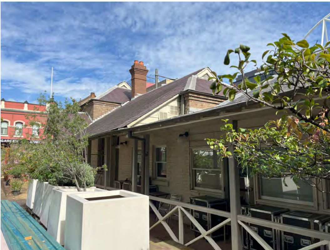
Figure 16 Rear (south) elevation of the 1980s addition (right) and the 1900-01 buildings (left)
