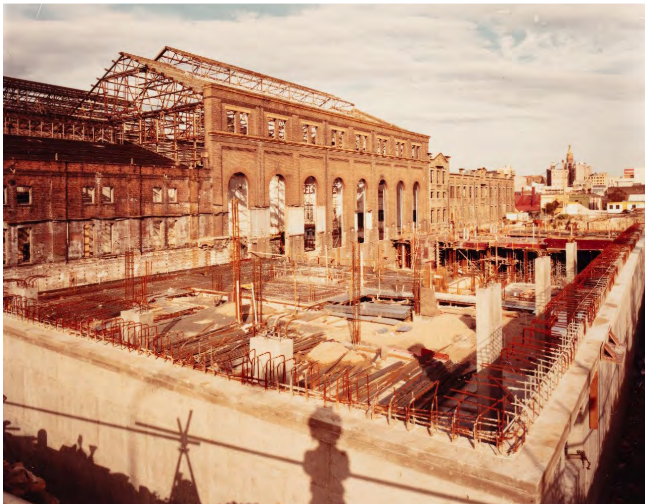
Figure 15 View looking south from the Post Office, c. mid-1980s: the footings of the Wran Building are in the foreground Source: Powerhouse Museum
