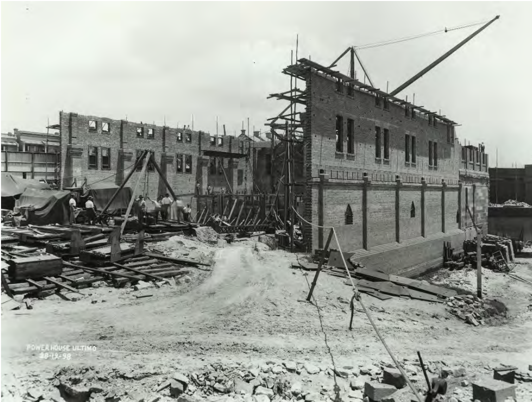
Figure 6 Power House under construction, 1898: the Engine House and North Annexe Source: NSW State Archives, NRS- 4481-2-[4/8645]- 122
