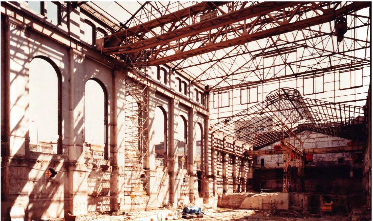
Figure 13 View looking north from the Turbine Hall, during adaptive works (1980s) Source: Powerhouse Museum
