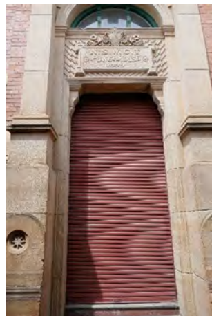
Figure 9 The original entry has been infilled with a roller door: note decorative spandrel panel
